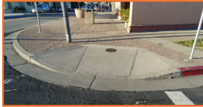
Existing Ramp without Detectable Warning
