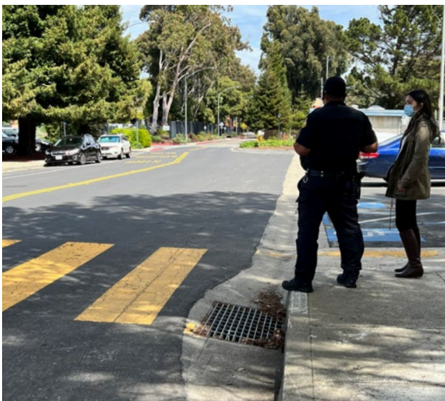
Figure 17. A view of the storm drain that prevents construction of a curb ramp on the south end of the crosswalk.
