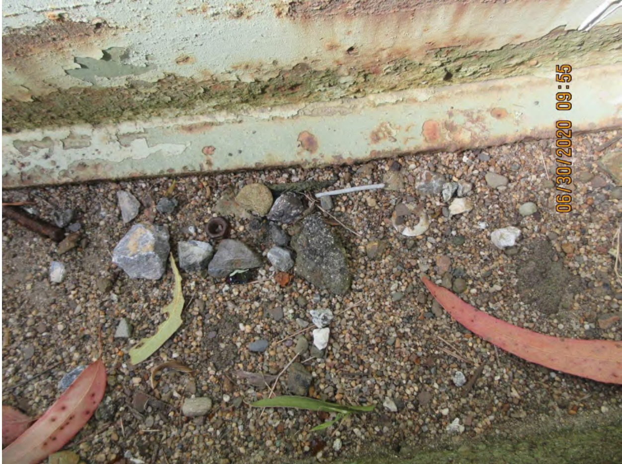
Photo 12: Tank 10 - Rusting Around Perimeter of Tank Bottom
