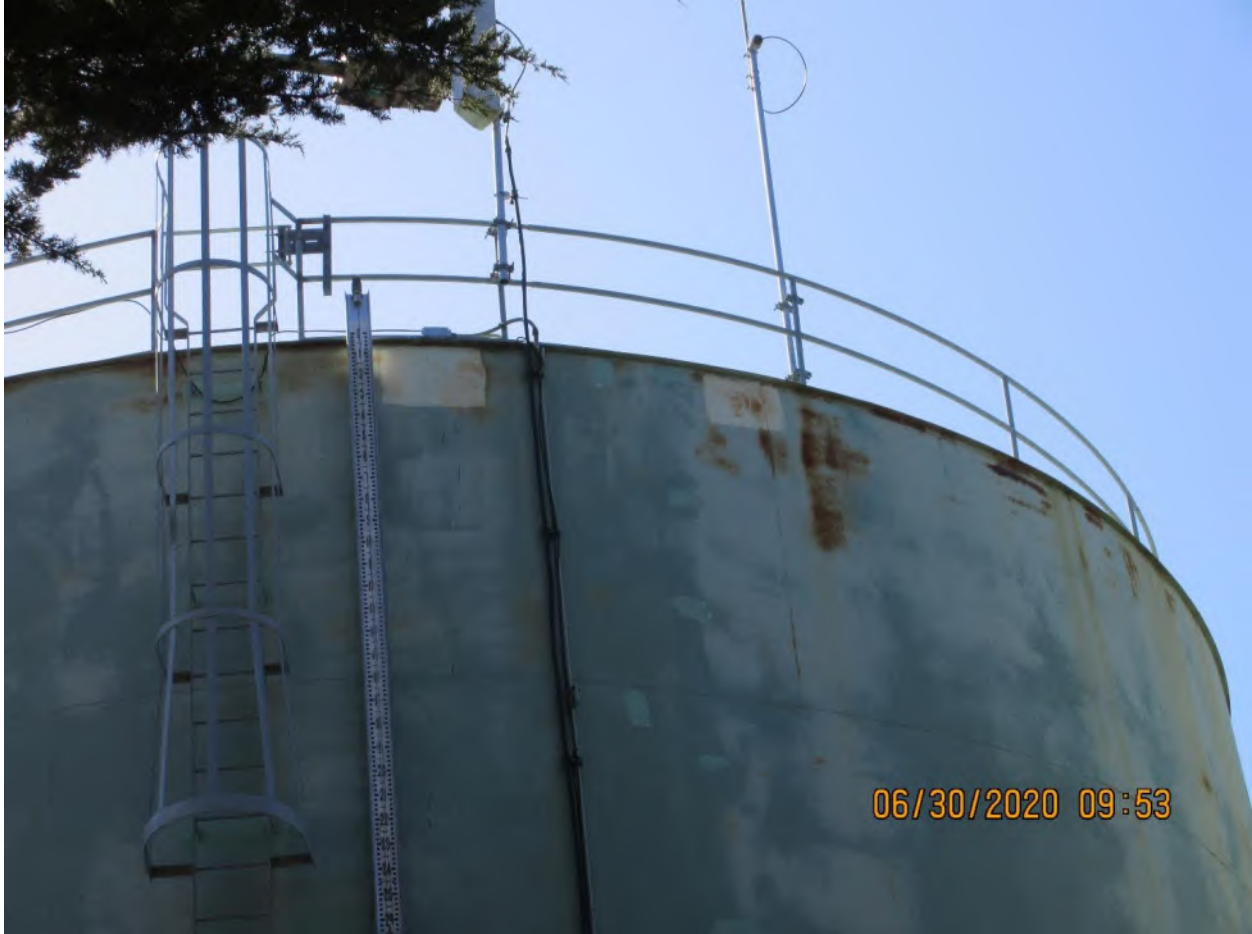
Photo 11: Tank 9 - Rusting Around Perimeter of Tank
