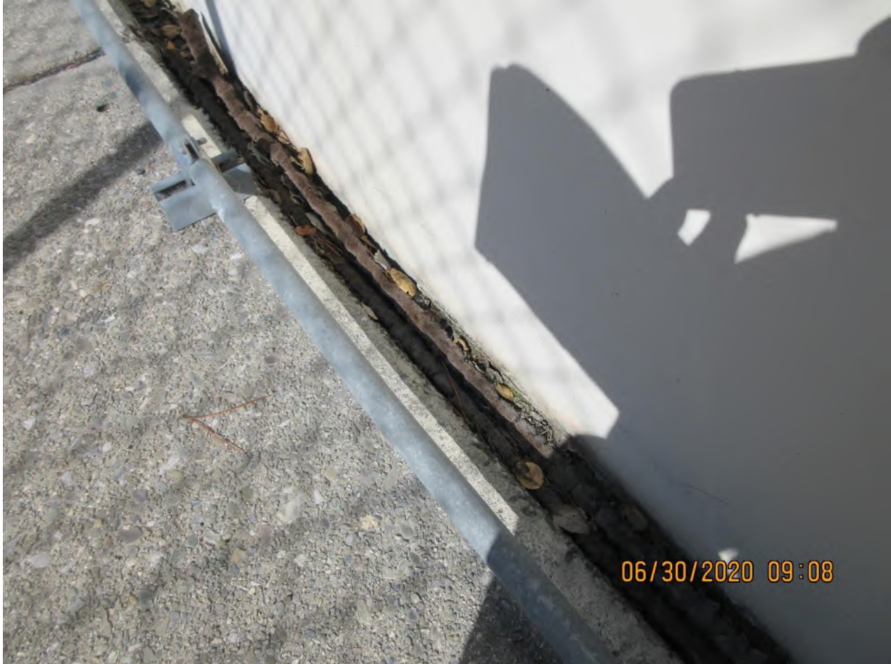
Photo 3: Tank 4 - Deteriorated Caulking Around Tank Shell
