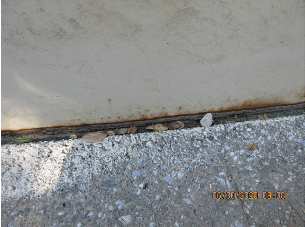
Photo 4: Tank 4 - Minor Rusting At Base of Tank
