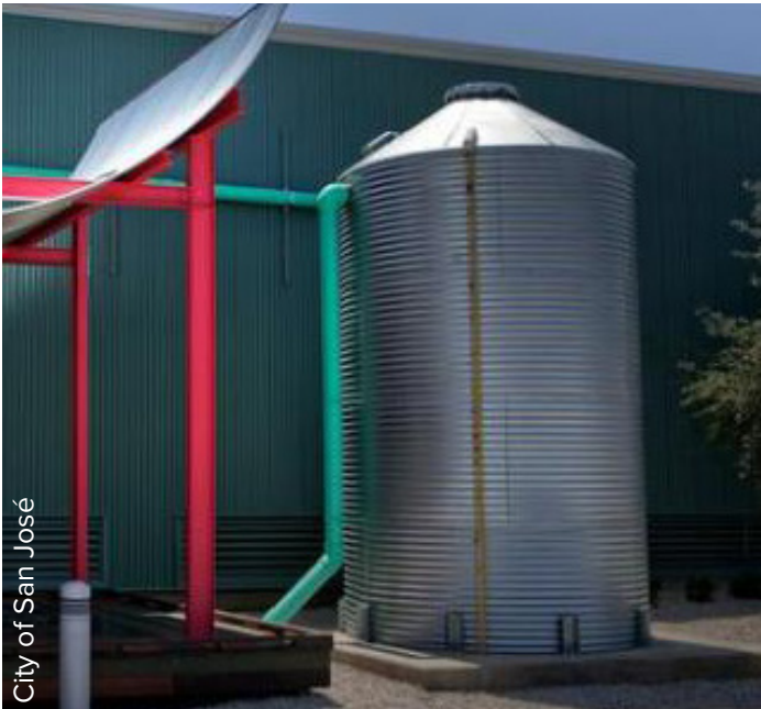
Rainwater Harvesting Cistern - Environmental Innovation Center, San José
